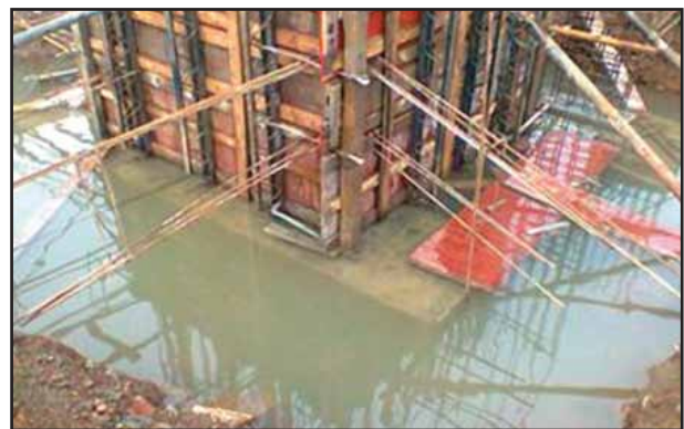
Fig 4: Anti wash-out concrete had set properly within 24 hours and work on further lifts could start immediately
