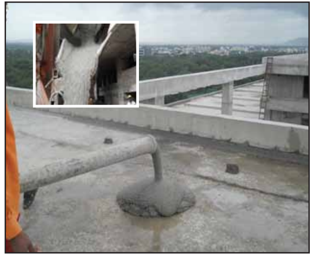
Fig 3 Elitecrete™ is a low-density, free-flowing concrete used for thermal insulation purpose for a commercial building in Pune (Inset-Elitecrete™ being unloaded)
